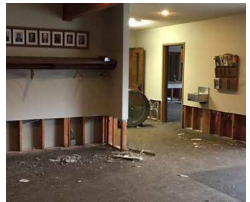
Damaged carpet, woodwork, and drywall were among the repairs faced by Sumas (Wash.) CRC after flood waters receded in early December 2021.
