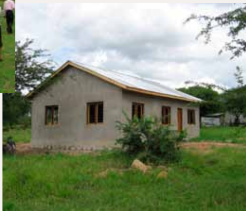
This is one of three houses built by the community to attract teachers.
