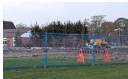
Demolition equipment and fencing remained around the former site of the Holland Marsh District Christian School after the building's demolition in November 2023. Holland Marsh CRC rises in the background.
