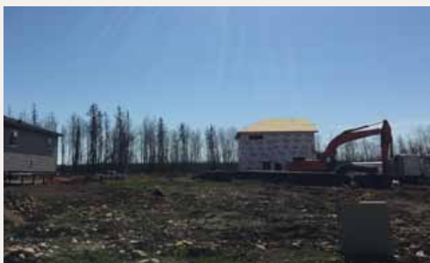
This house, destroyed by a wildfire, will be rebuilt this summer with the help of World Renew volunteers.
