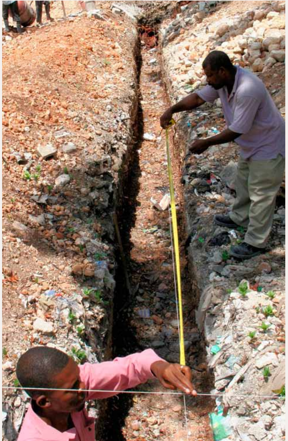
Pastor Elihu Metallus, foreman, and Edouarnis Estivil, project manager, measure the foundation for the new Jacquet church in Haiti.
